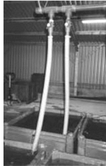
Flexible feed pipes and control valves
