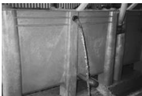
Seawater outlet pipe
